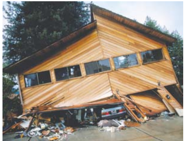
This home in the Santa Cruz Mountains collapsed in the Loma Prieta earthquake. (Photo courtesy of USGS)
