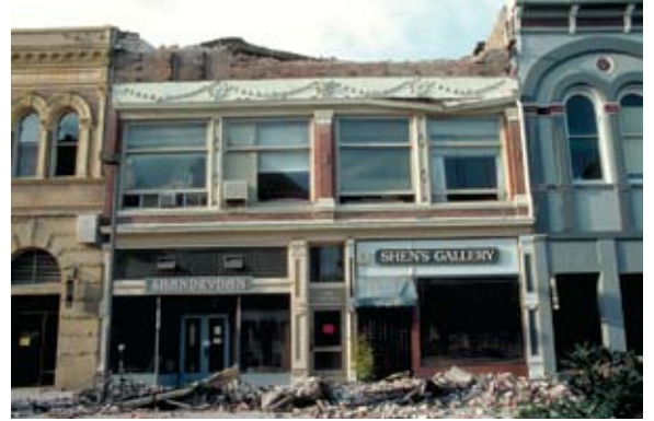
These small businesses in Santa Cruz, California, were heavily damaged in the 1989 magnitude 6.9 Loma Prieta earthquake, but both eventually reopened. (Photo courtesy of USGS)
