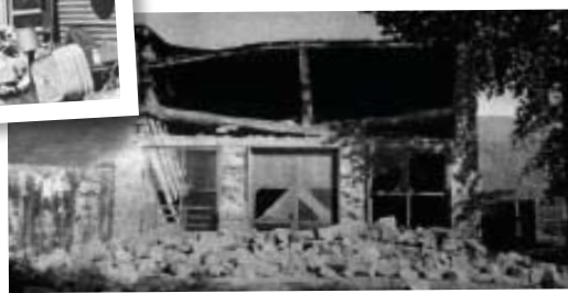
Smaller photos: Damage caused by the M 5.7 Richmond (Cache Valley) earthquake of 1962 (top) and the M 6 Elsinore, Utah, earthquakes of 1921 (bottom). (Photos courtesy of, respectively, Ariel D. Benson, Richmond, Utah, and the F. J. Pack Collection, Special Collections Department, University of Utah Libraries)
